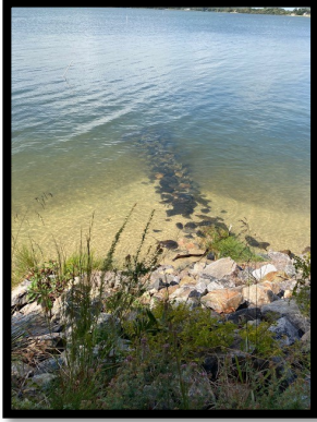
This reinforced shoreline of riprap revetment and groins has held up since Isabelle.
